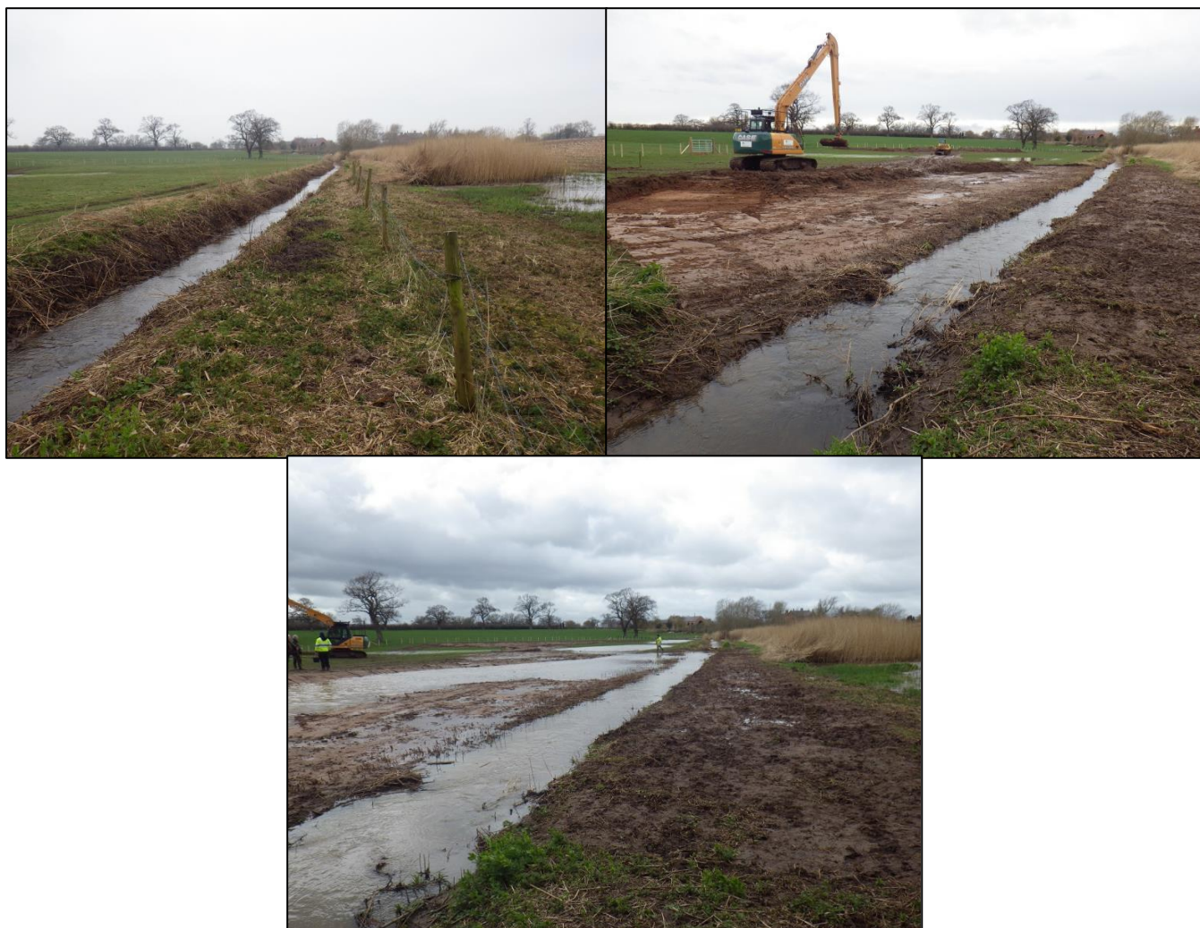
Figure 5-7 Floodplain restoration (pre-construction, during construction and completion) as part of the Mill Brook project (UK) (Source: amended from Environment Agency for EA WWNP case studies)
