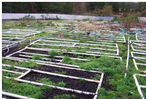
Plate 3.5 Peat puraflow filter bed. The pipes should be covered to prevent the effluent being washed away with surface run-off during heavy rain. Photo by Dr Julie Fossitt
