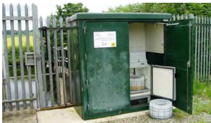
Figure 1: the 24-bottle refrigerated autosampler housed in its kiosk on the banks of the River Derg next to the Derg water treatment works.
